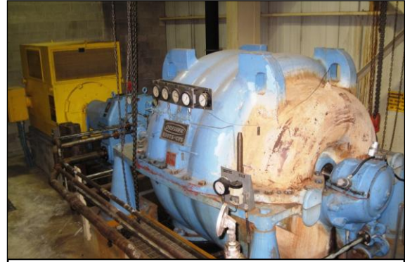
Vacuum system issues also apply to exhauster systems
