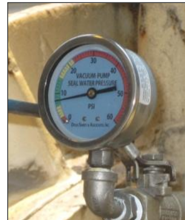
Accurate seal water pressure measurement is important
