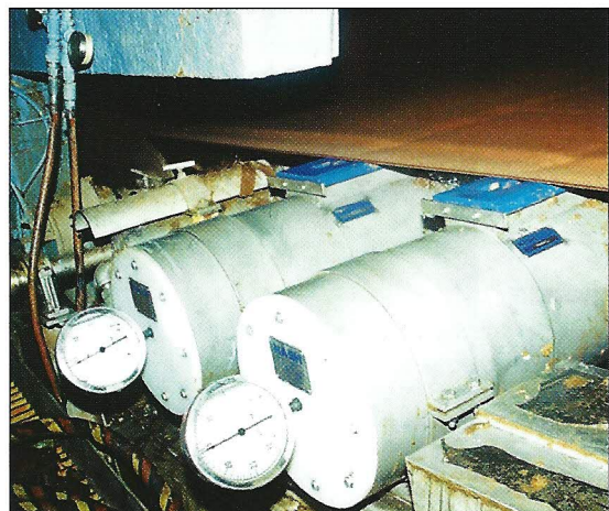
It is important to locate vacuum gauges at the suction box or roll as shown on these uhle boxes.
